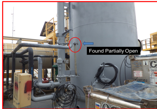
Sight Glass Gauge Cock found partially open during a Performance Based Risk Inspection
