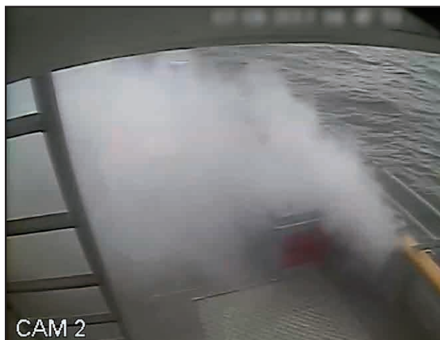
Figure 2: Fire extinguishing powder billowing from the natural air vent
