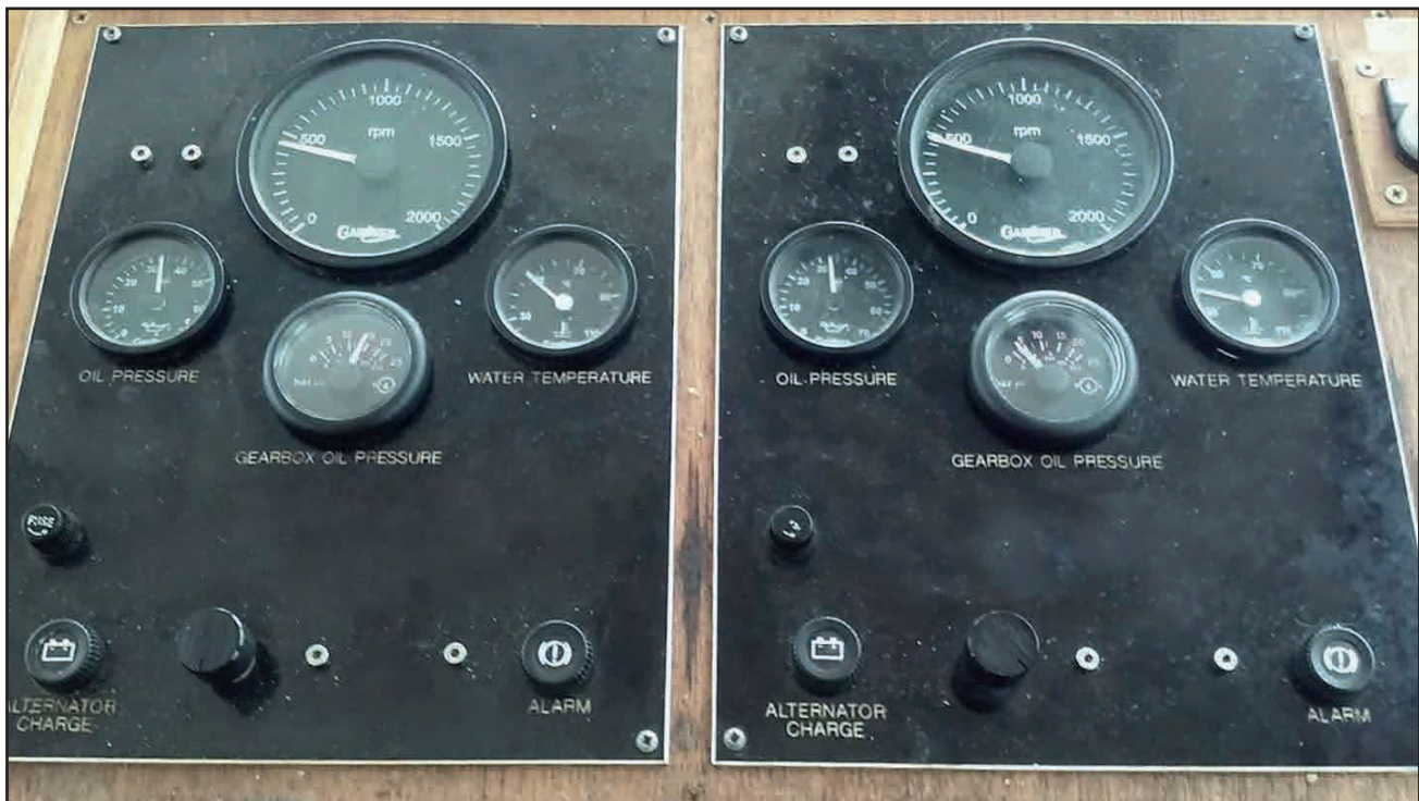
Figure 2: The wheelhouse console
