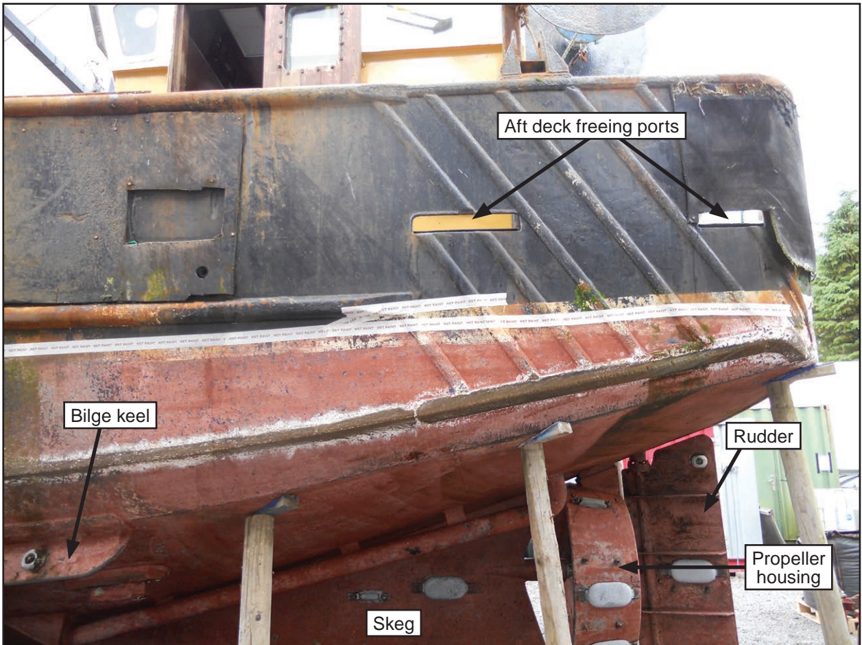
Figure 12: Pre-purchase survey – hull form aft end port side showing aft skleg design
