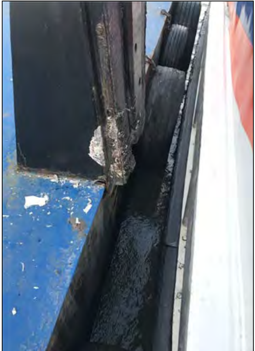
Figure 1: Damage to pontoon
