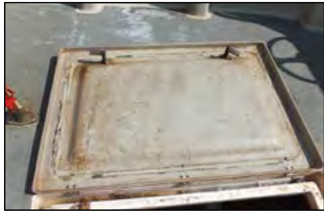
Figure 2: Missing hatch seal
