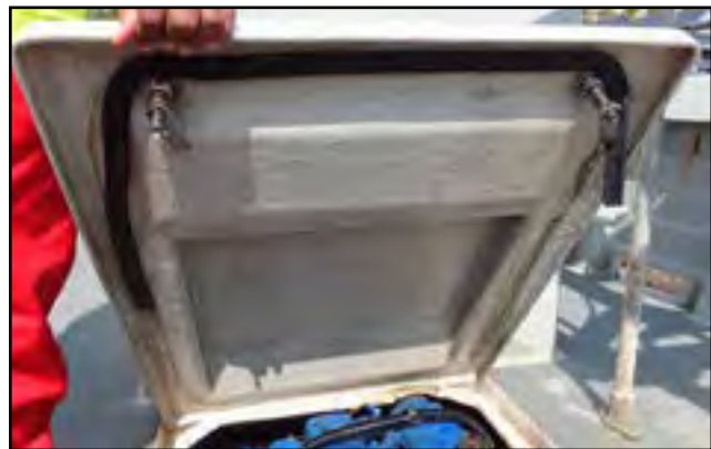
Figure 3: Damaged hatch seal
