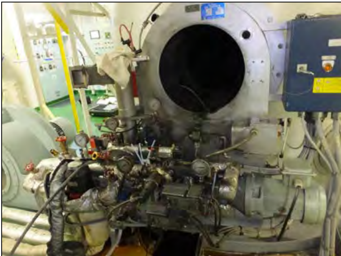
Figure 1: The damaged boiler
