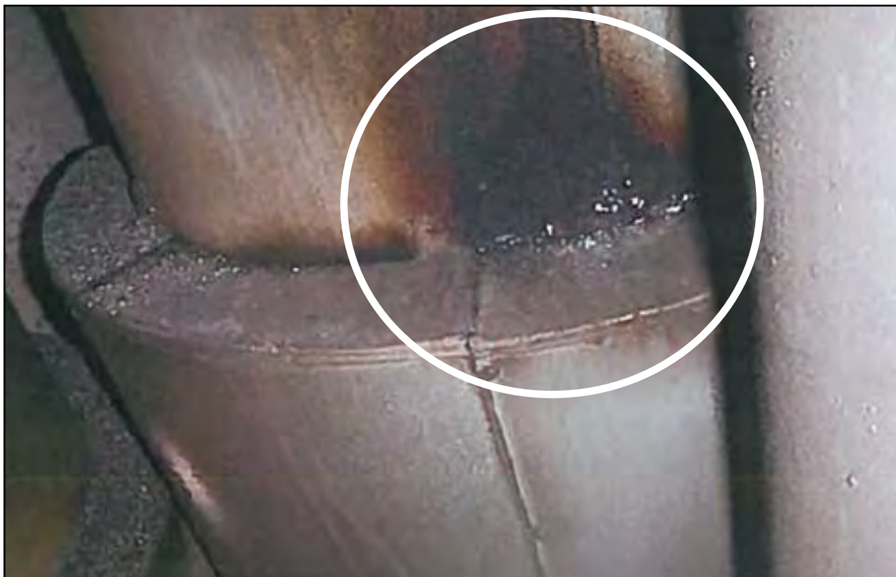
Figure 2: Damaged area of exhaust lagging
