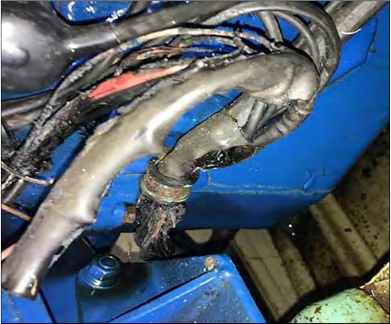
Figure 2: Heat damage to electrical cabling
