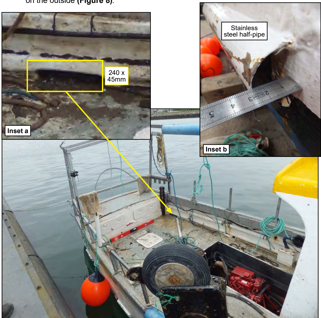
Figure 8: Freeing ports (inset a: enlarged view and inset b: stainless steel half-pipe fitted on the hull outside)
