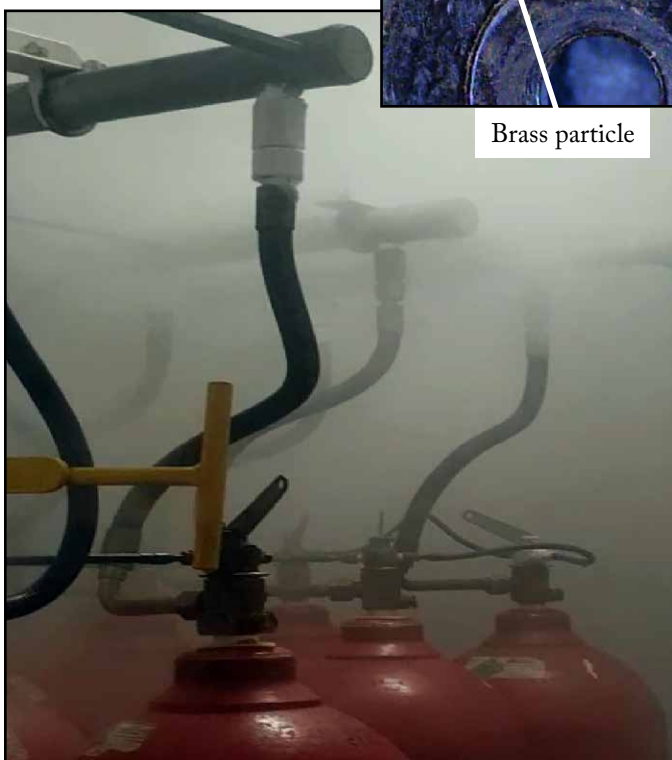
Figure 1: CO 2 leakage (inset: brass particles embedded in cylinder valve seat causing it to leak)
