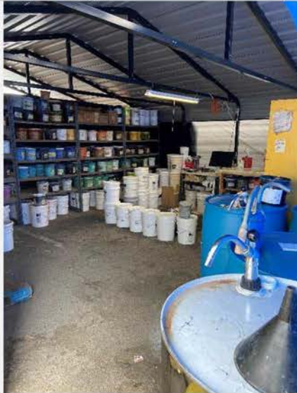
1: Finding 1, Chemical Storage with no fire extinguisher
