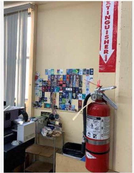
6: Photos of Fire Safety Equipment
