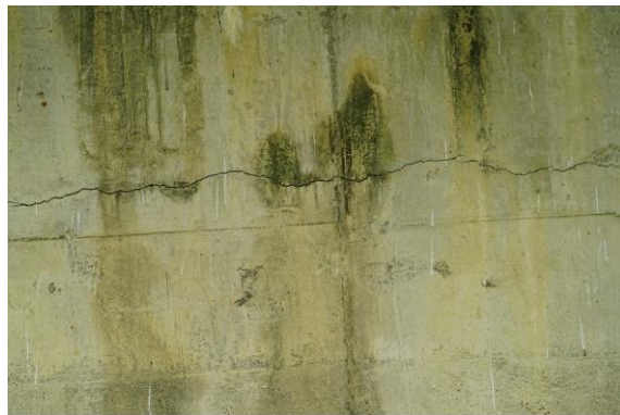
Figure 15. Crack image case 2
