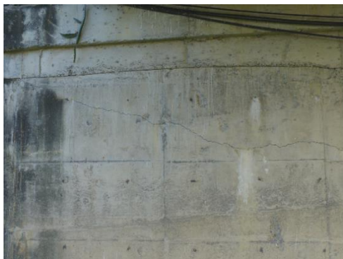
Figure 11. Crack image case 1
