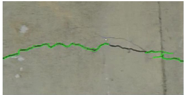
Figure 23. A broken crack.
