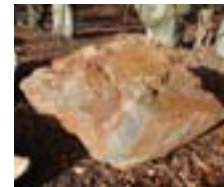
Slate with rust
