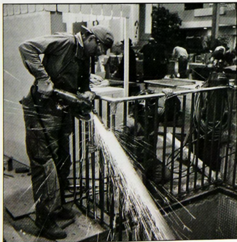
A welder puts finishing touches on the Midtown Plaza Mall. The entire Midtown Plaza complex, including the 18-story Tower, encompassed seven and a half acres of shopping and business space.
