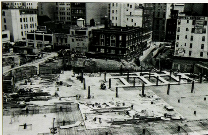
Ground was broken on April 6, 1959. This image, taken in Spring 1961, shows construction of the underground garage.
