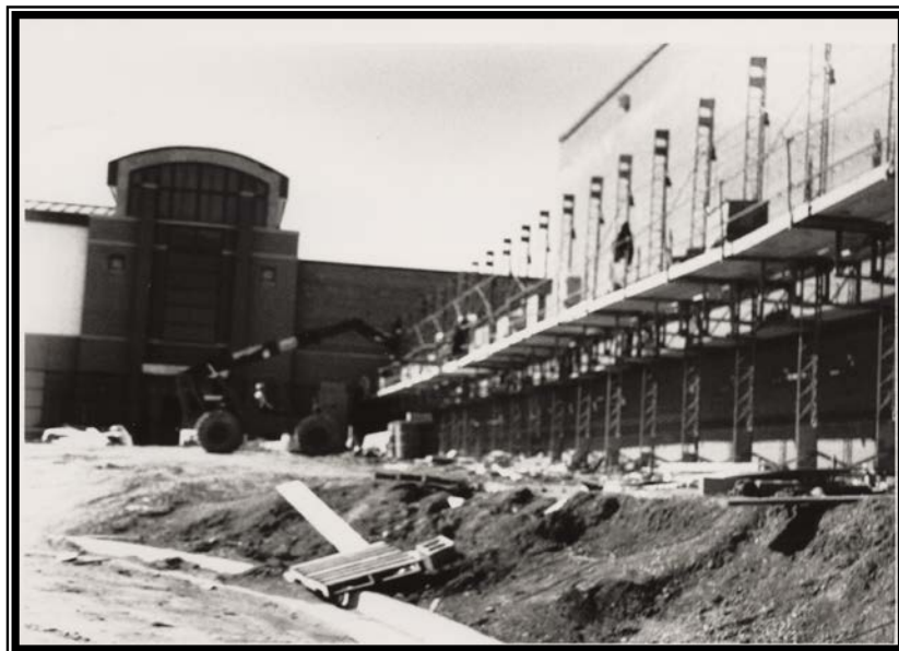
Figure 17. Emerald City (now the Robert J. Dole Community Center) under construction sometime in 1993.
