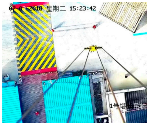
Figure 6. A sample image taken by the tower crane camera at the construction site.
