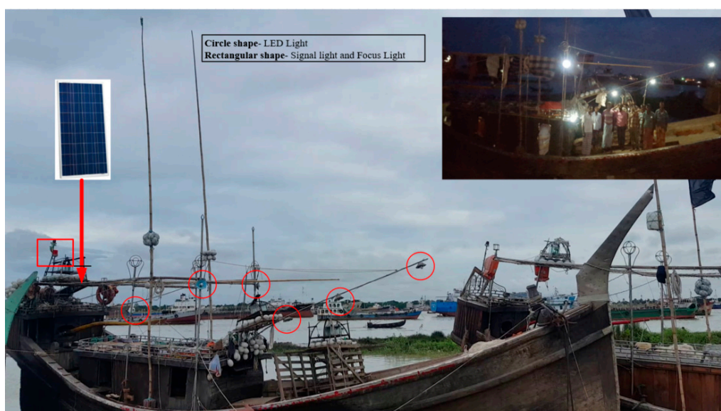
Figure 12. Full view of the fishing trawler on which the proposed system is installed, and in the inset, the night view of the fishing trawler is given after the project implementation.
