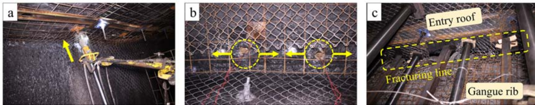
Figure 16. Test processes of the DRF technique. (a) Drilling fracturing holes; (b) Charging with energy binding tubes; (c) Roof fracturing effects.
