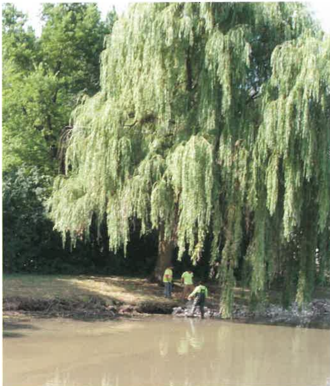
This photo shows Wilderness Pond South shoreline being lined with rip rap by Fremont Township Highway staff. Observe the significant erosion and sediment suspended in the water. This shoreline was repaired in 2018 during this SMC WMB grant by Fremont Township and MPRD to help prevent sediment flowing into Diamond Lake. Photo by Tori Trauscht.
