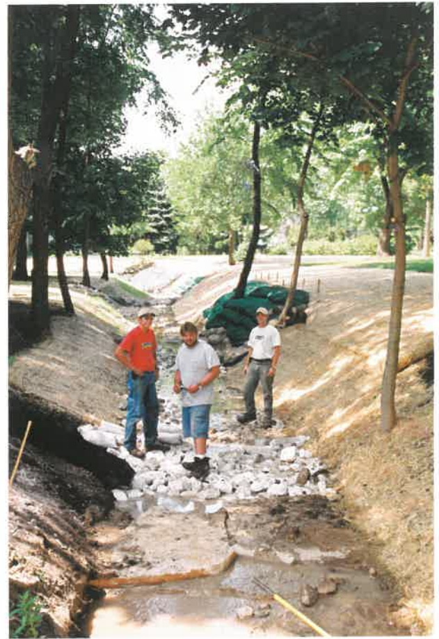
Contractors used BMPs such as rock, erosion control fabric and native seed to restore this section of West Shore Park in 2005. Photo by Tori Trauscht.
