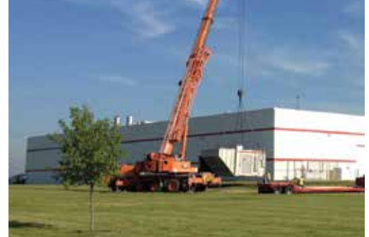
Pre-fabricated Containerized Test Cells
