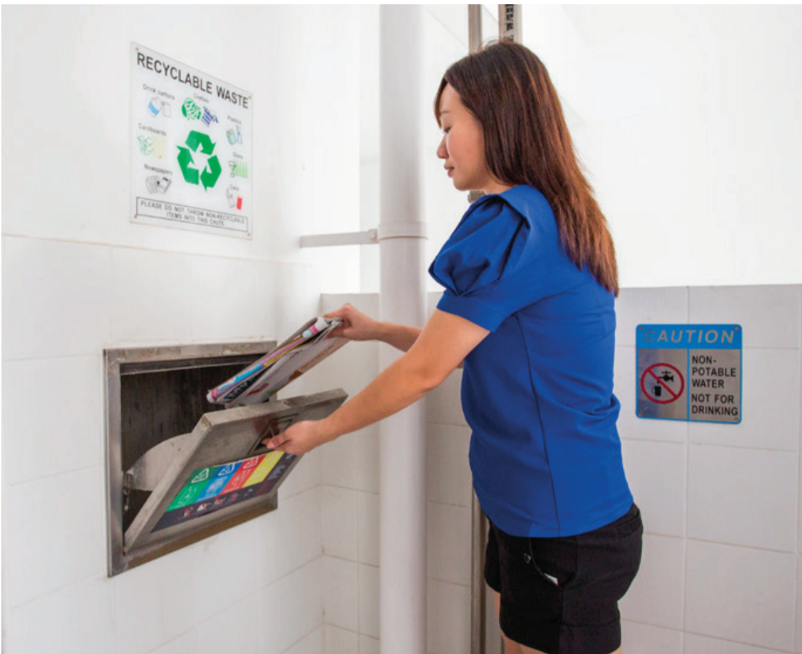
Separate chutes for recyclable waste
