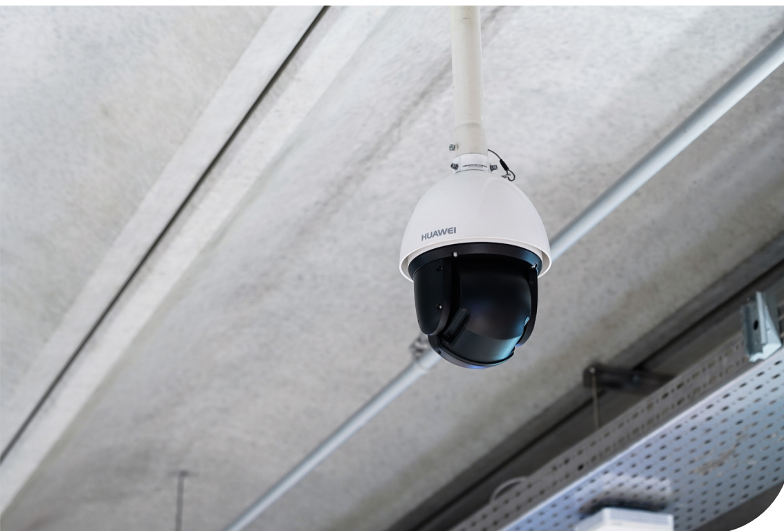
A Huawei CCTV camera installed in Suvarnabhumi Airport in Bangkok, Thailand.
