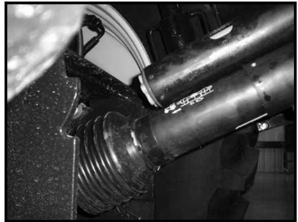
Shown Properly Cut To Length With Plastic Guard Tubes In Place
