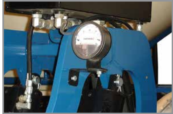
ASD system pressure gauge
