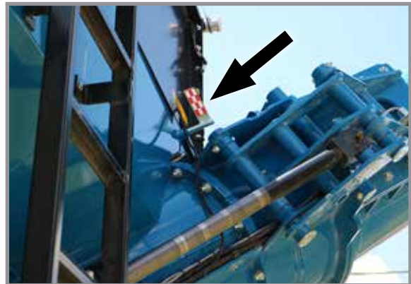
Flow Gate Position Indicator
