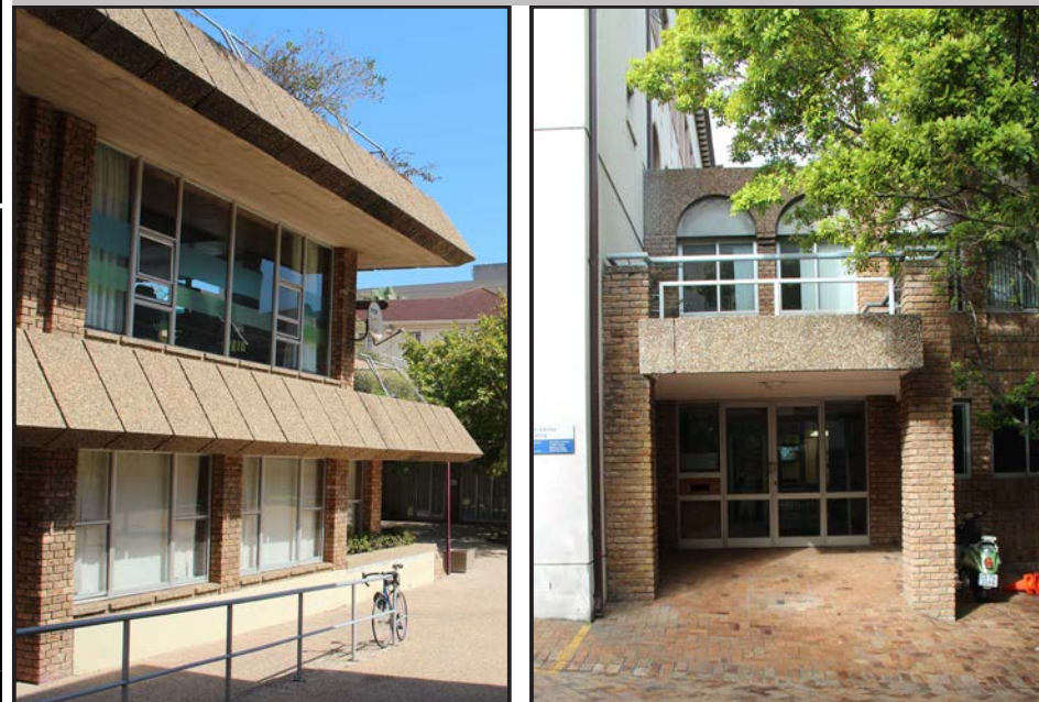
Image: Detail of the textured aggregate panels (L) and junction of old and new buildings (R).
