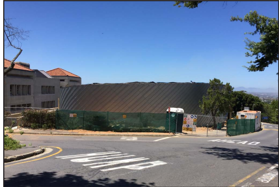
Image: New Lecture Theatre, still under construction, as seen from Ring Road/Madiba Circle.
