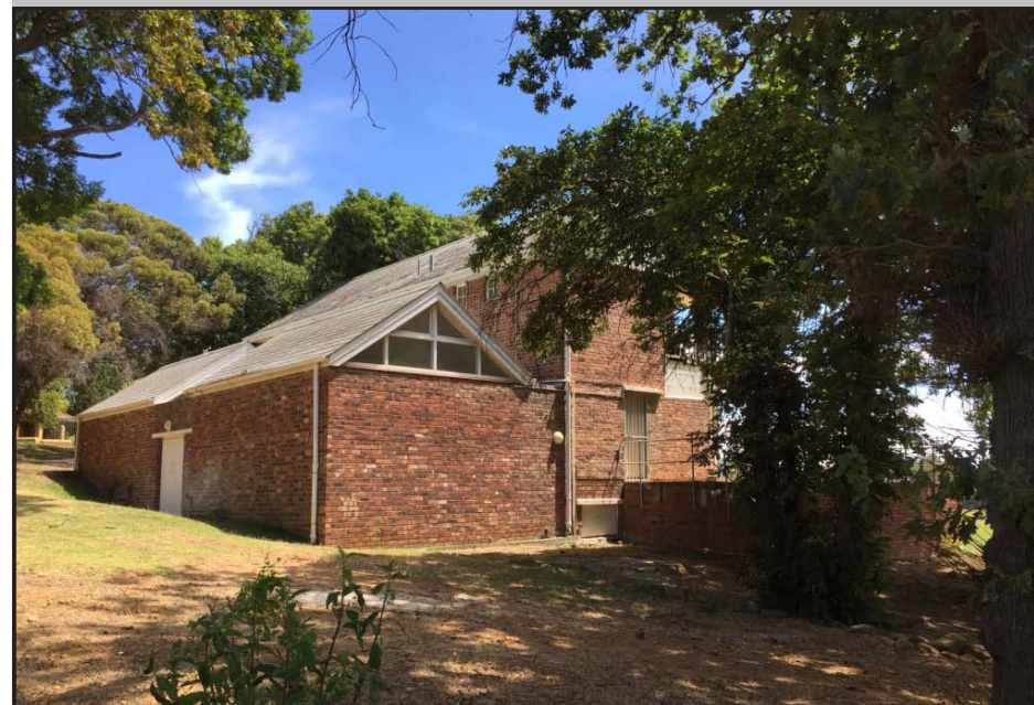
Image: View of the south-east facade of the building as seen from the approach from Bremner Access Road.
