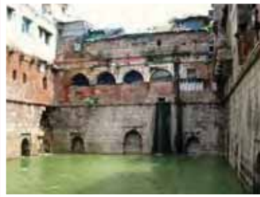
Baoli wall collapsed in July 2008
