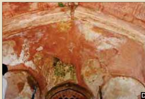
A,B and D :Alcoves before conservation works.The cement patches were applied to the alcoves in 1960's
