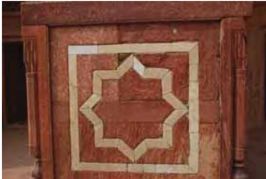
Condition assesment of the stones of the lower facade of Humayun's Tomb
