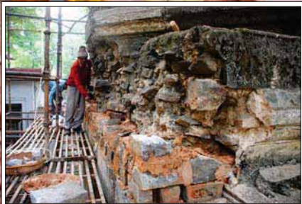
▲ Missing masonry at parapet level required to be re-built
