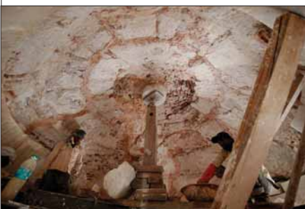
▲ Stone carvers fix the repaired marble elements back to their original location on the structure
