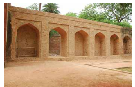
▲ Collapsed portions of the enclosure wall were reconstructed using traditional materials and techniques
