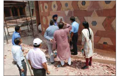
▲ The Core Committee reviews stone repairs and replacement undertaken on the neck of the dome at Humayun's Tomb. Master craftsmen have used traditional tools and craft skills to prepare stones for portions that had deteriorated beyond repair.
