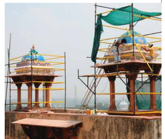
Conservation works at Humayun's Tomb, such as repairing the sandstone platform (top), replacing 20th century cement flooring with original stone paving (centre) and restoring glazed tiles to the canopies (bottom) are carried out by craftsmen using traditional tools, materials and building techniques.
