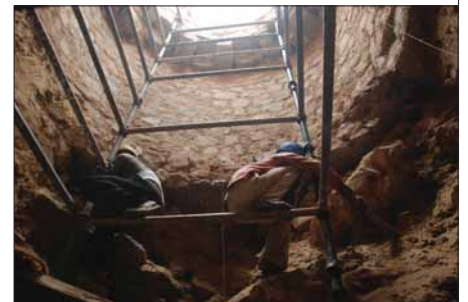
▲ De-silting of historic wells in the project area, and removing decades of rubble and deposits from them
