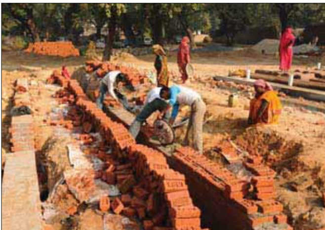
(Below) Civil works in progress of creating parking space in Batashewala Complex
