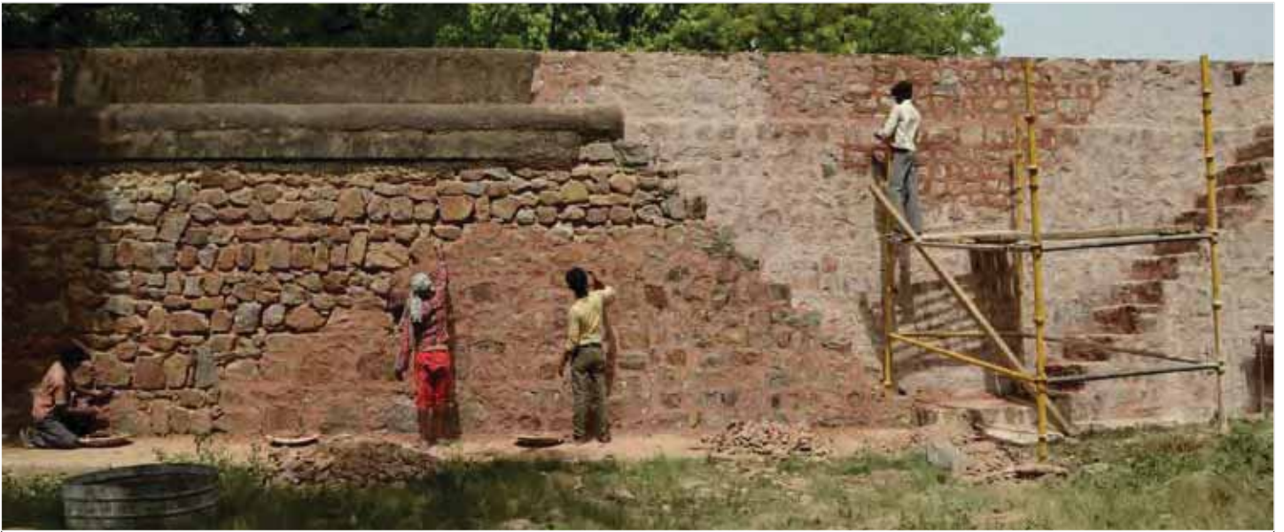
(Above) Removal of dead cement pointing and stitching the cracks in the enclosure wall and bastion chambers was followed by pointing with lime mortar.
