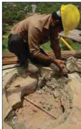
Craftsmen use hand tools to remove deteriorated wooden section and cement concrete laid here during a past 20 th century repair
