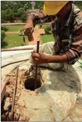
Water entered the vessels and was retained due to the cement that was applied over the marble surface of outer dome in the late 20 th century
