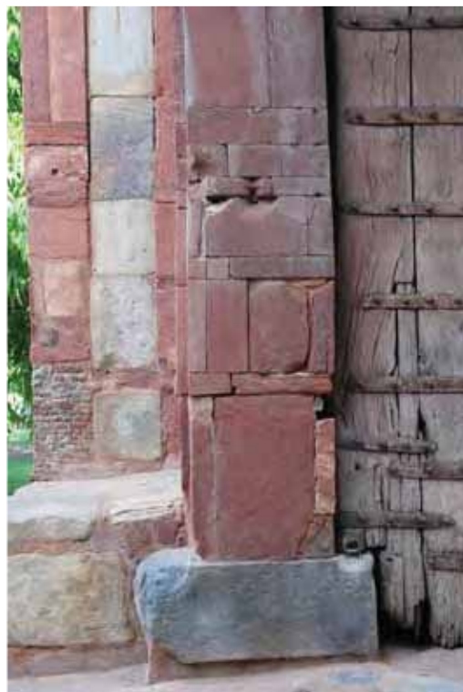
(Right) Following a stone-by-stone documentation, decayed sandstone was replaced by new stone pieces by carefully matching the original.
