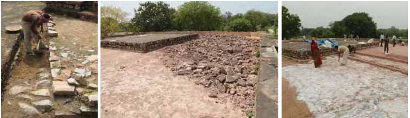
(Left) Dismantling existing cement concrete from flooring; and (Middle) terrace and (Right) laying lime concrete. The final phase of conservation works at Sundarwala Mahal are supported by HUDCO through NCF
