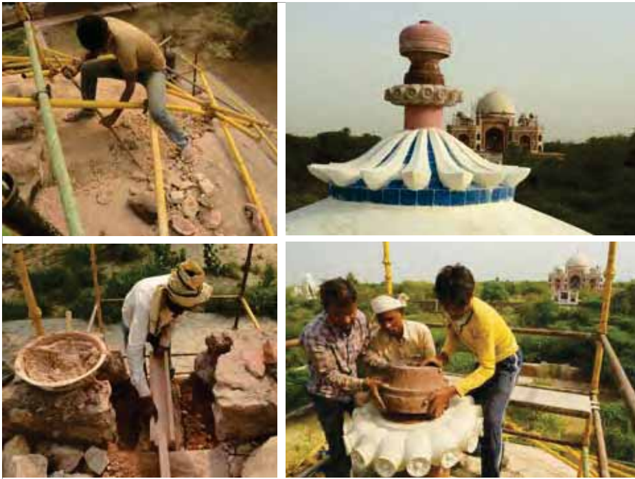
Broken portions of the finial were found collapsed on the roof. Master craftsmen prepared matching finial pieces to restore on finial on the dome.
