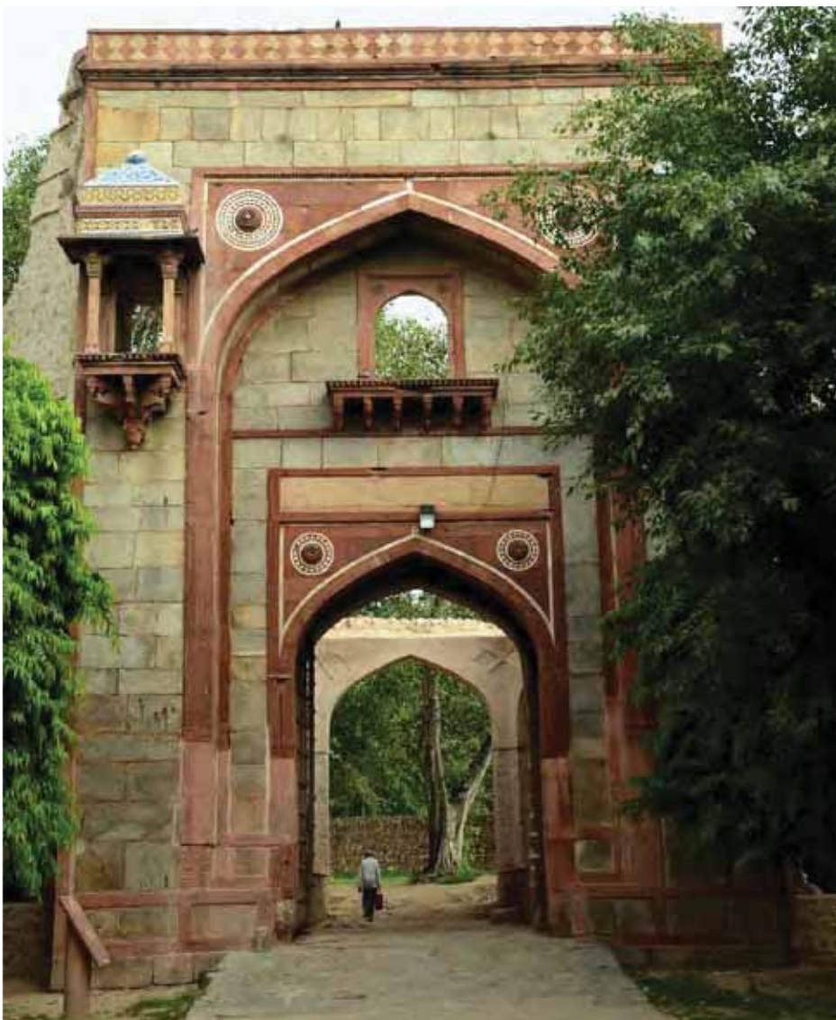
Arab Serai Gateway: after conservation. Conservation works on the Arab Serai Gateway were undertaken with a grant from the German Embassy .
