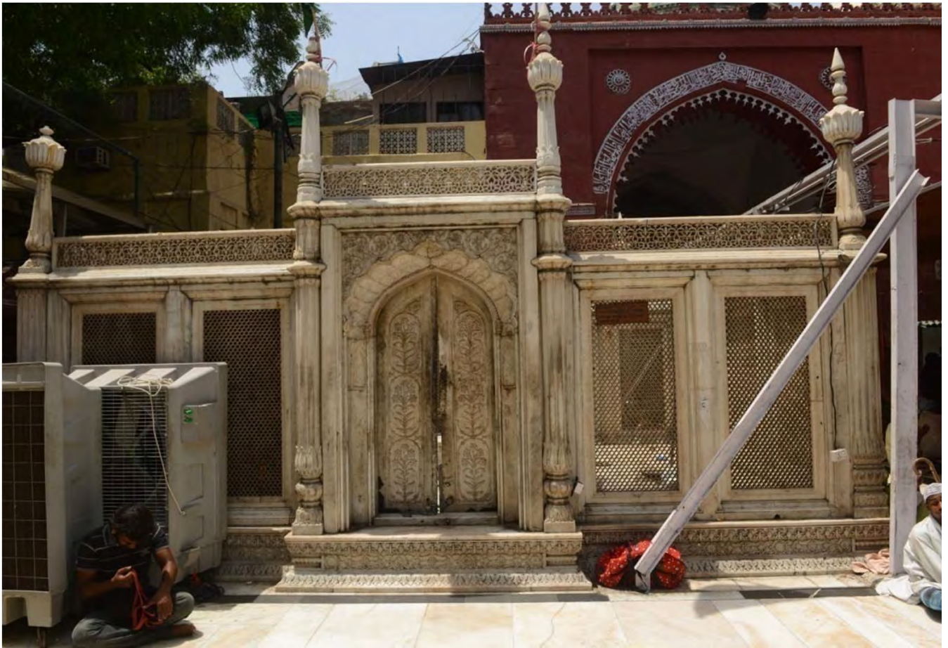
Unplanned architectural fittings are a major threat to the original architectural element.
