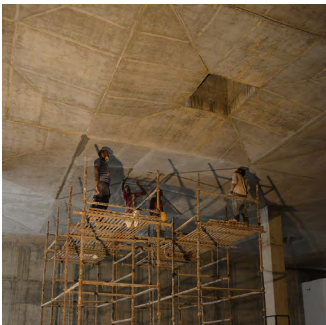
Rendering of exposed concrete finish ceiling Cutting of 10mm groove in the pleated ceiling of gallery block.
