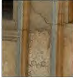
Missing patterns and cracks
