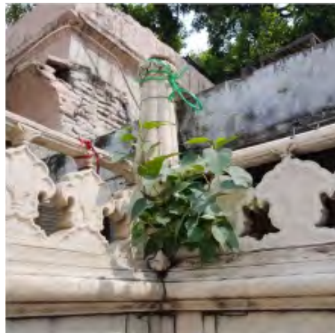
Damaged marble pinnacle
