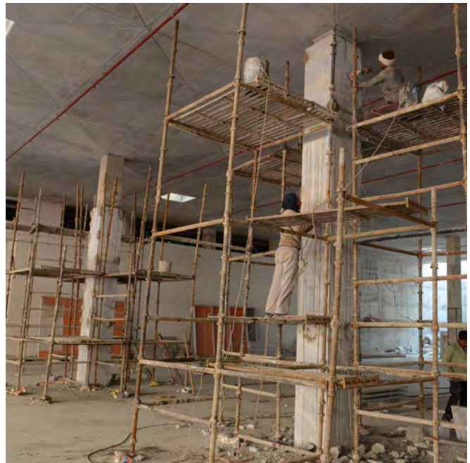
40mm thick white marble cladding on the columns of main exhibition gallery.
