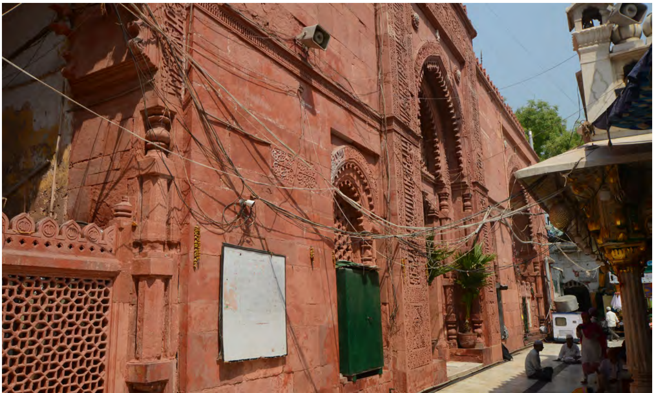
Before and After images of Jamaat Khana mosque where layers of paint were removed to reveal the original sandstone facade.
