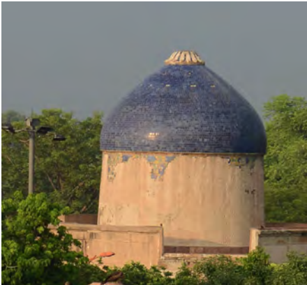
Missing tile work on the finial of the dome being restored with tiles matching the original
