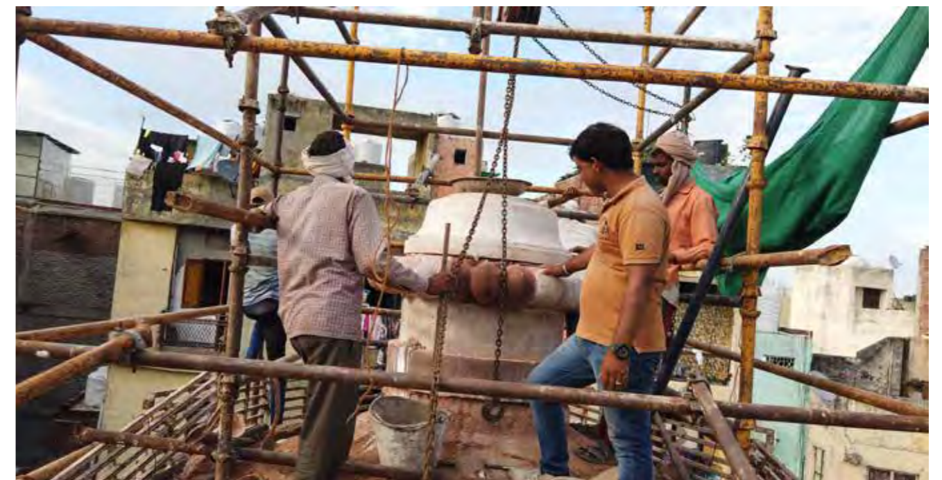
The damaged finial has been secured for display at the museum and a replica matching the original was restored to the dome
