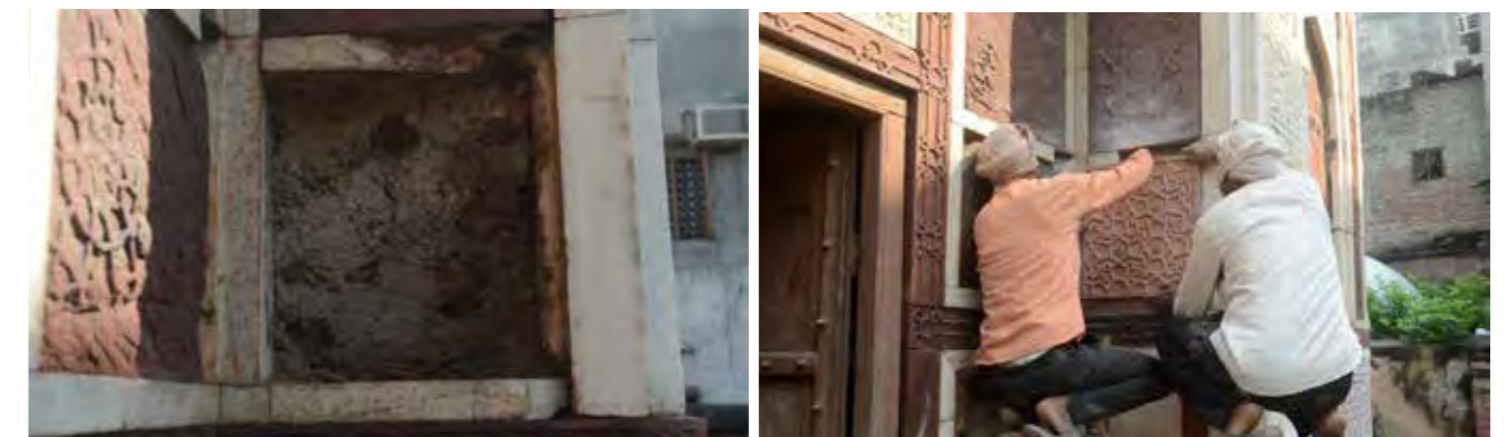
(Left) Some of the intricately carved stone slabs had deteriorated beyond repair and (Right) were replaced.
