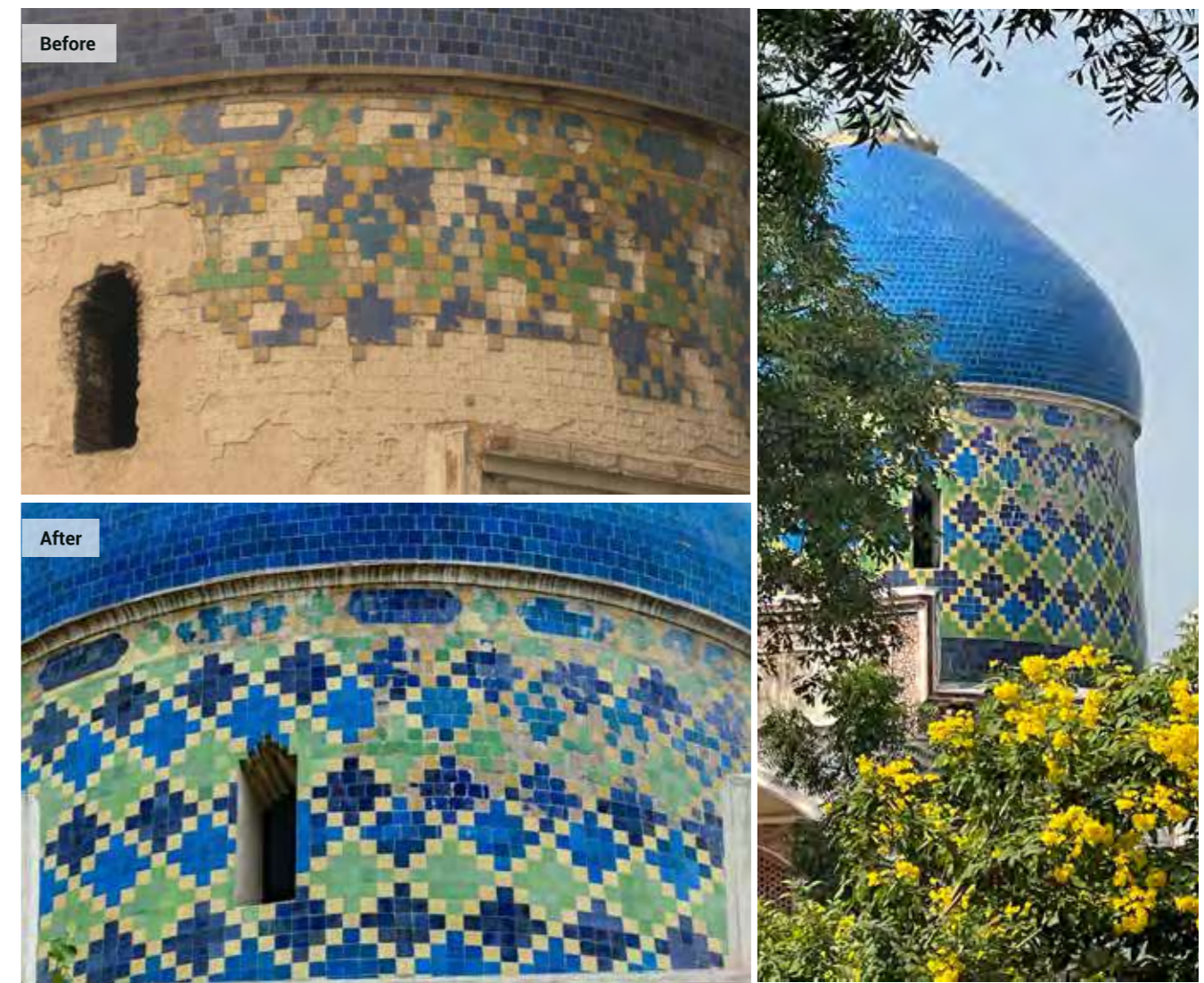
Missing tiles were restored as per the original pattern. The restoration of the tile work was important to prevent further loss from the neck and to restore the continuous geometric pattern formed through the arrangement of the four distinct colours found here
