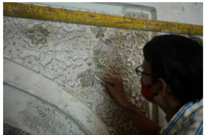
(Left) Lime plastering of the walls by craftsmen providing provisions for electrical conduits and switch board points; (Right) Careful cleaning of the ornamental plaster work on the ceiling.
