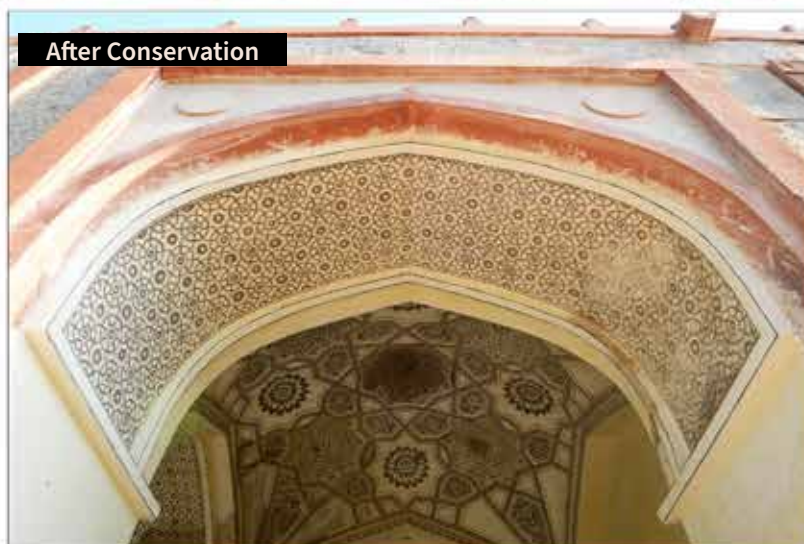
(Above) The chambers in the ground level arcade carries unique designs and ornamentation which were carefully restored where missing
