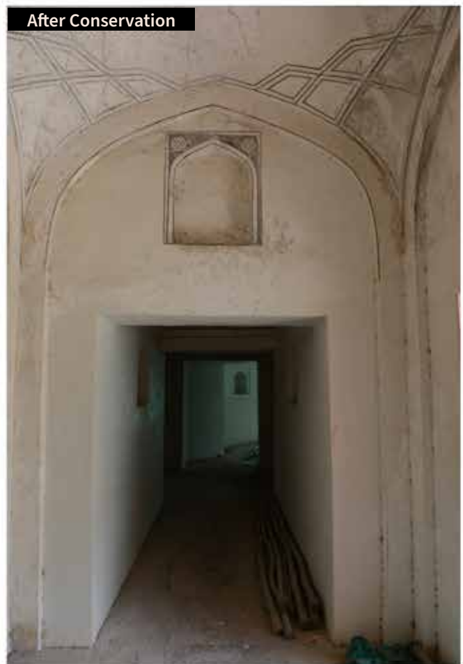
(Above) Deep cracks in the masonry were repaired using traditional methods and lime wash and soot layers carefully removed
