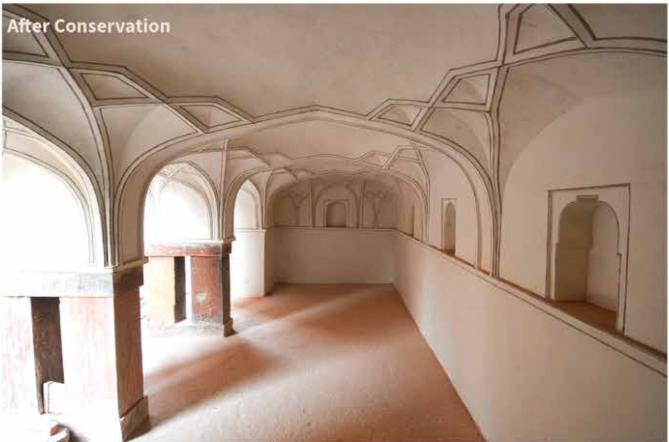
(Above) Water percolation from the roof above has been addressed to prevent further water ingress. The vaulted interiors have been restored using traditional craftsmanship.
