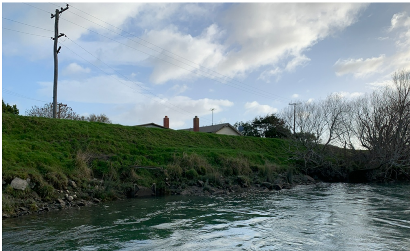
Figure 15: Erosion damage and slumping at Factory Road site, Paretai (March 2020).
