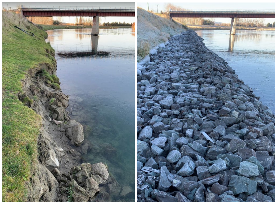
Figure 11: Riverbank Road floodbank at bridge near Stirling (LC21), before(left) and after (right) reshaping and vegetation stabilisation.
