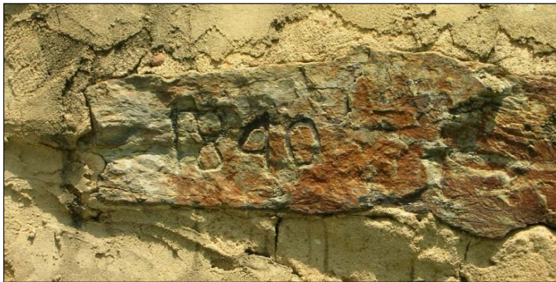
Figure 13. ca. 1840 date-inscribed chimney attached to the south elevation of the Strayhorn-Blackwood House.
