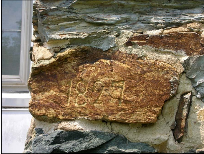
Figure 12. ca. 1827 date-inscribed chimney attached to the south elevation of the Strayhorn-Blackwood House.
