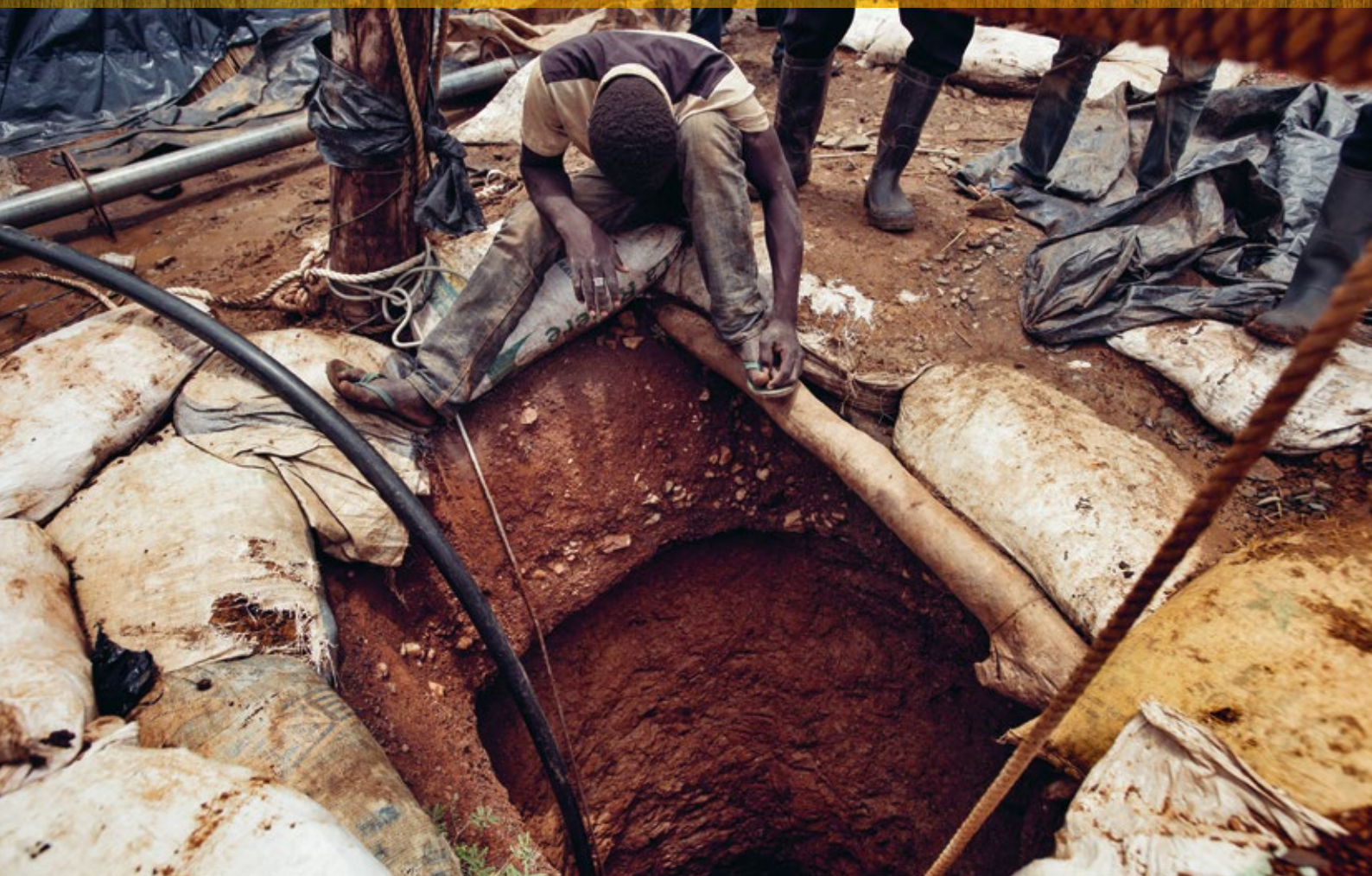
Diggers wait their turn to descend into the darkness. Sandbags and wooden poles are makeshift measures to reinforce the shaft walls, up to 170 m deep. // Tikando mine site, 13th August 2015.
