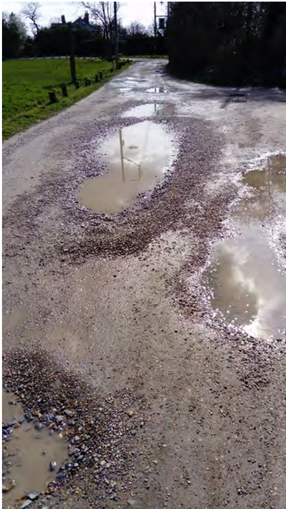
Figure 1 – Erosion on main through route
