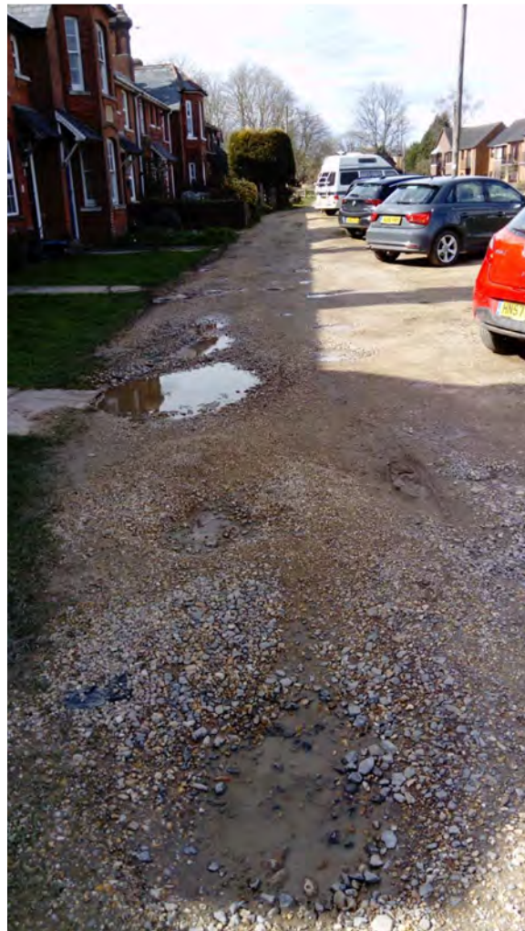
Figure 2 – Erosion at Bickerley Terrace
