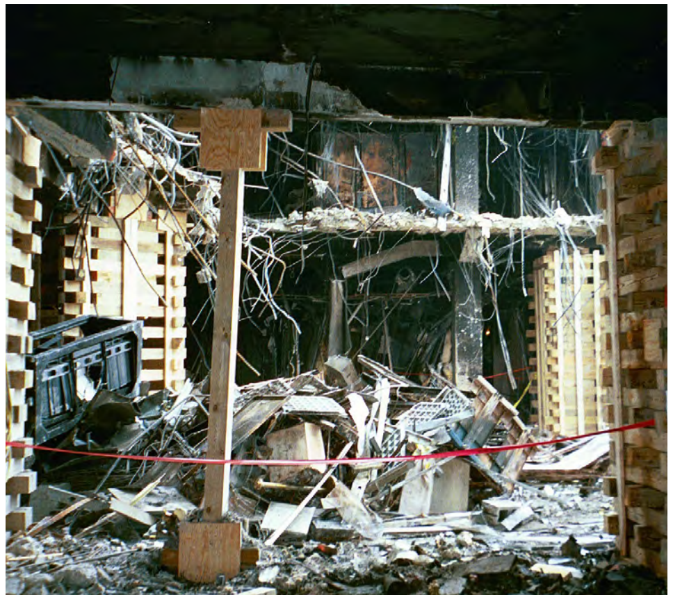
STRUCTURAL STABILIZATION — Before the team could begin its recovery work in earnest, Pentagon walls and ceilings had to be safely stabilized.
