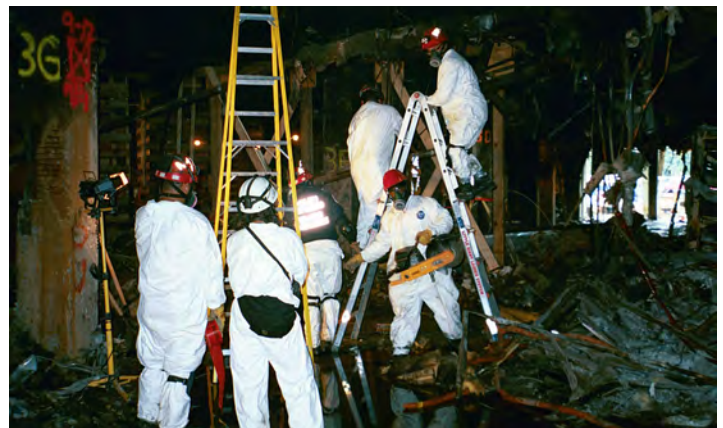
INTEGRATED TEAM — Members of New Mexico Task Force-1 team work together to safely shore up portions of the Pentagon while sifting through and removing debris.
