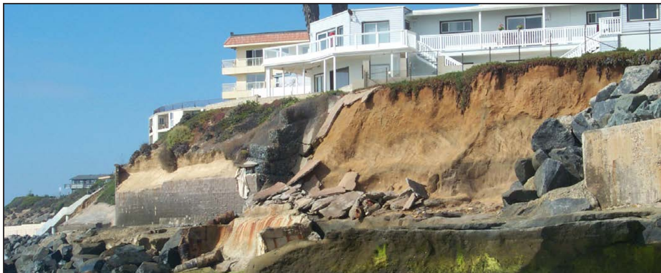
Erosion has become a major issue in the community. Tidal erosion can have a major effect on residential areas along the coast.
