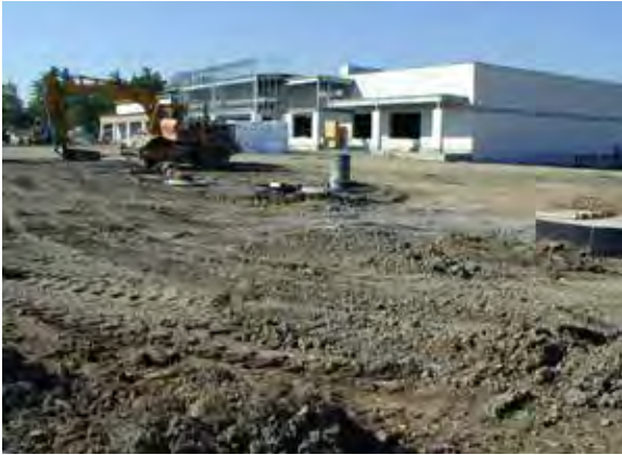
Figure 22.2. Construction activities cause bare compacted soil with potential for water and wind erosion, and challenges with revegetation.
