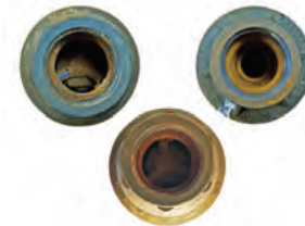
Inlet and outlet of worn pressure regulators.
