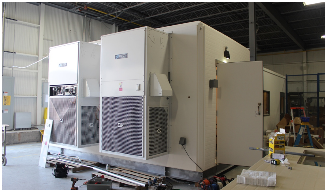
Wall-mounted air conditioning units
