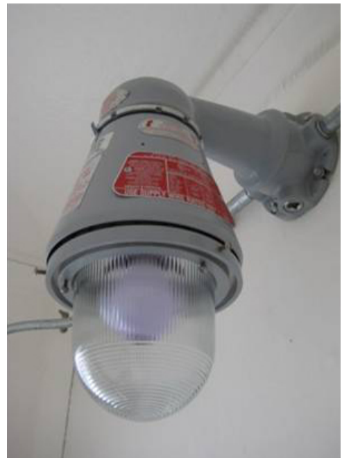
An explosion-proof fluorescent light
