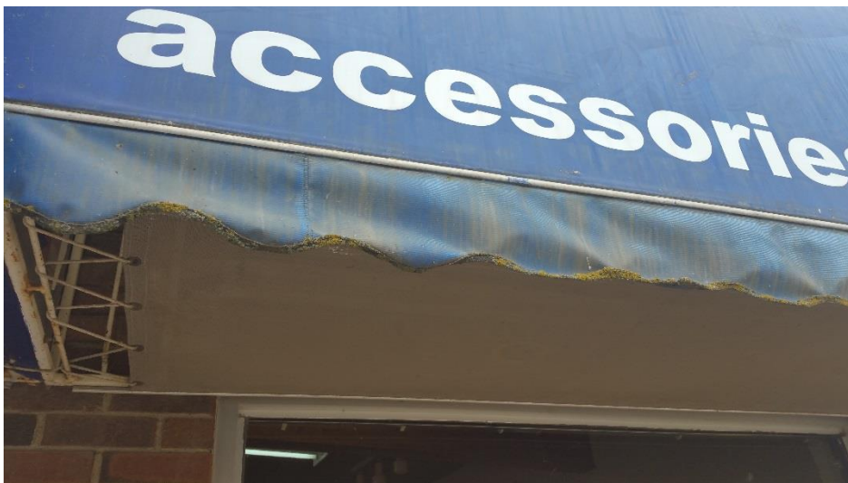
Figure 16: This awning over a storefront is in need of repair.
