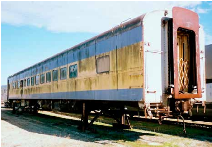
Prior to rebuilding, Ringling crews set a passenger car up on jackstands so that workers can access the undercarriage and the interior to move the work along. Rhett Coates
