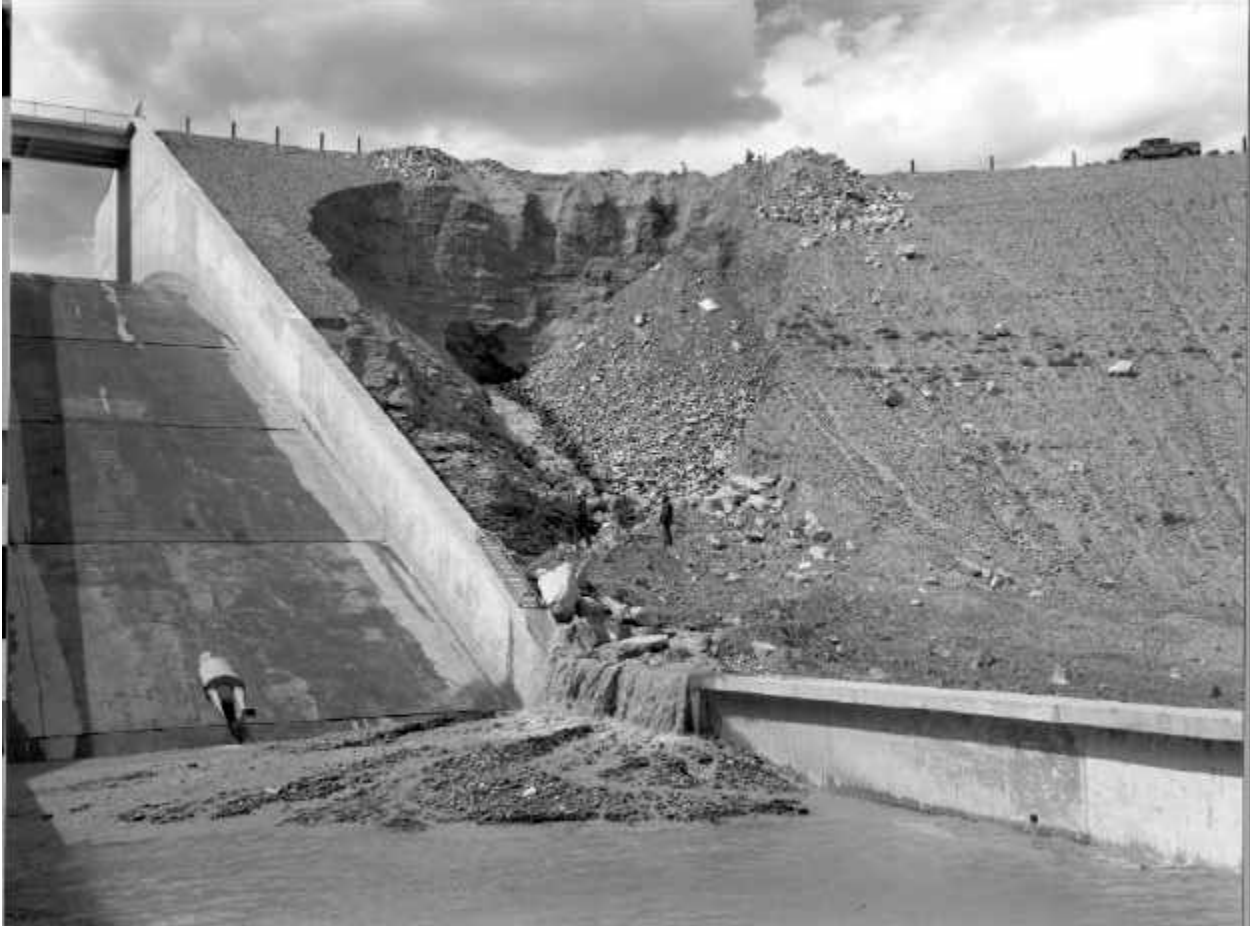
Figure 12 - Fontenelle Dam - Large Sinkhole on Downstream Slope
