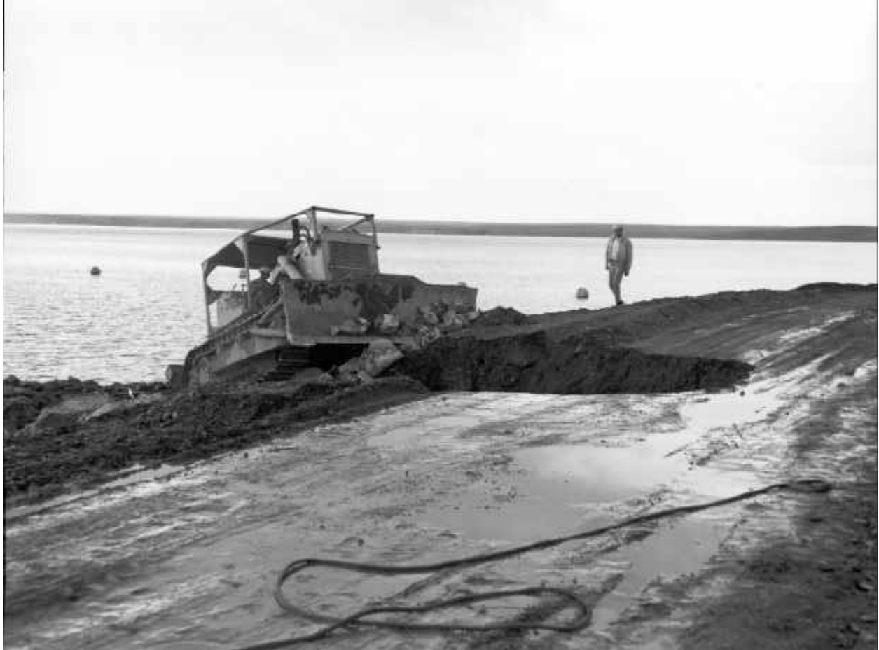
Figure 13 - Fontenelle Dam - Crest Sinkhole
