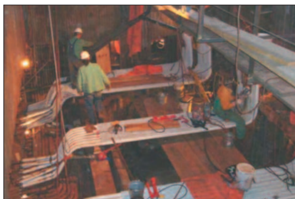
Figure 15 Steam loop at Niles PCC plant (Viswanathan, 2008b)
