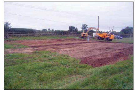
Plate 5: Stripped barn footprint and area of hard standing viewed from north east
