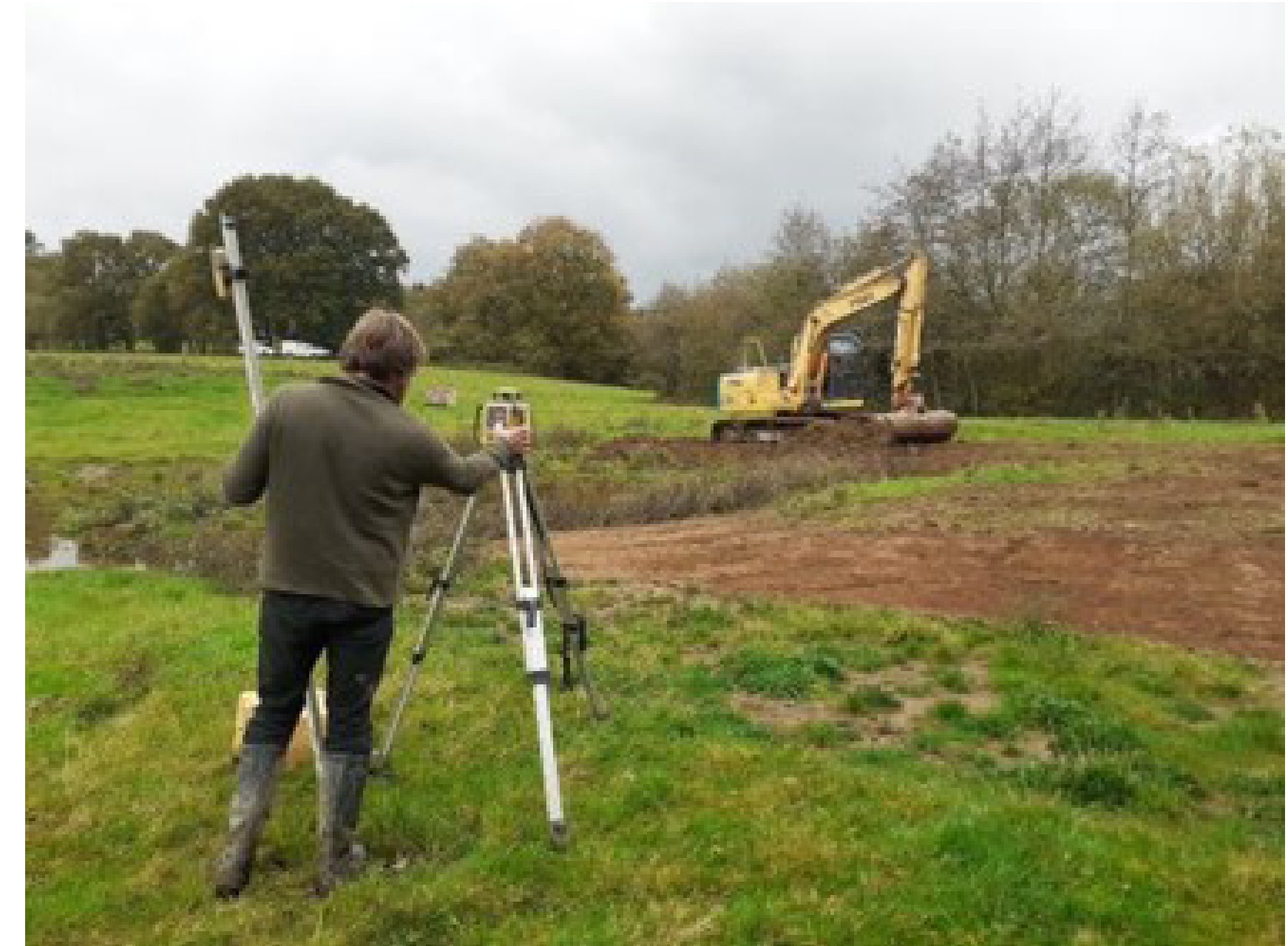
Working with contractors to put in water attenuation features in the landscape – these work as adaptations for both flooding and drought scenarios – Sussex Wildlife Trust Wilder Landscapes Image © Sussex Wildlife Trust.
